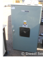
© Diesel Service & Supply
