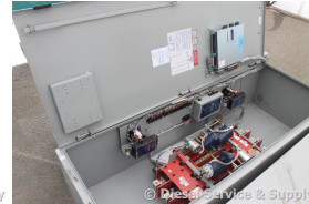
© Diesel Service & Supply
